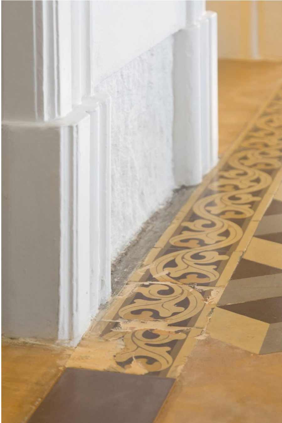
Fig. 4. Faulty hydraulic mosaic floor. Source: © ITS Ivo Tavares Studio
